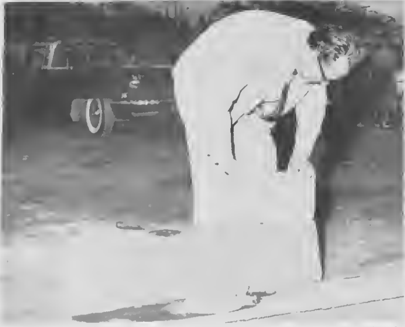
DEPUTY PORFIRIO Croes puts the first stone in place in the Noord sports center wall. This symbolic act underlined the long-range program of the Aruba Sports Union to build a series of athletic fields and facilities throughout the island.
